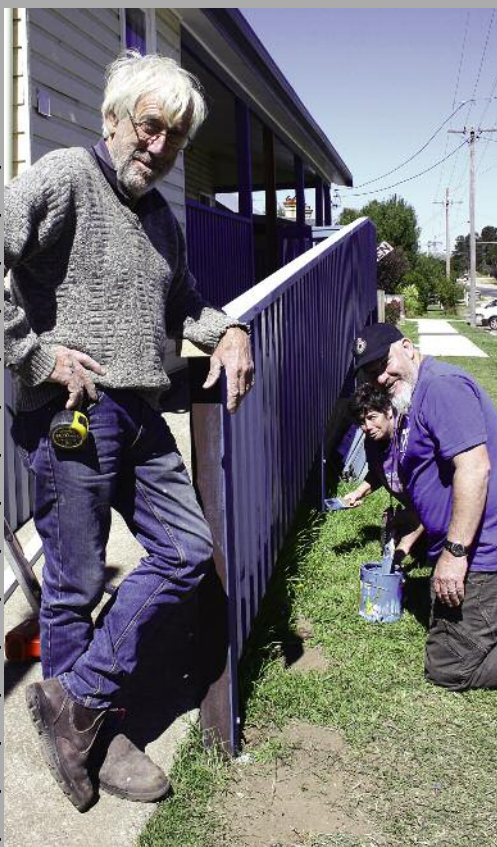
HANS VISSER, JULIE BAKER AND THEIR NEXT-DOOR NEIGHBOUR PUT THE FINISHING TOUCHES TO THE NEW DECK.
